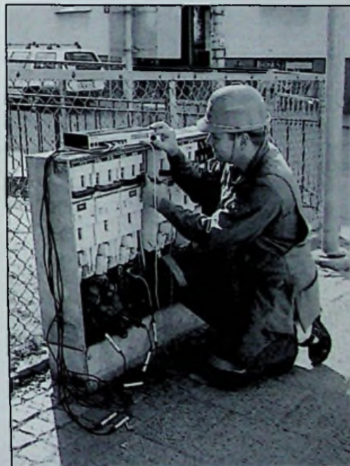
figuur 1: Meting on-site met Unipower DIP8000 Power Analyzer
